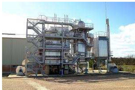
Figure 2. CIEMAT 3.5 MWth atmospheric bubbling fluidised bed facility
